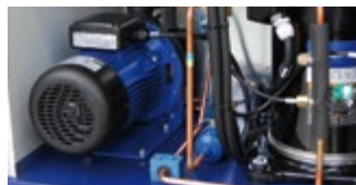
Pump P3 (3 barg) / P5 pump (5 barg, optional).
